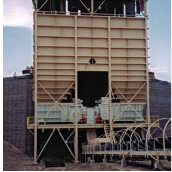
Two JOY Feeder-Breakers operating simultaneously at 2,000 TPH each.
