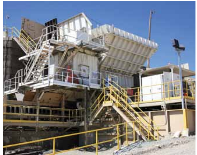
Skid mounted Feeder-Breaker with a 300 Ton hopper crushing phosphate ore to a minus 12 inch product size at 2,000 TPH.
