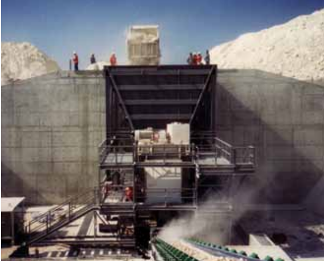
Fixed mounted Feeder-Breaker positioned beneath a 200 ton hopper receives ROM limestone and produces a minus 150 mm (6") product size at 700 MTPH.
