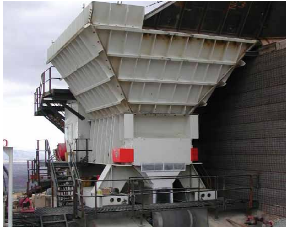
Feeder-Breaker crushes phosphate ore for conveyor belt transport at a rate of 2,000 TPH.
